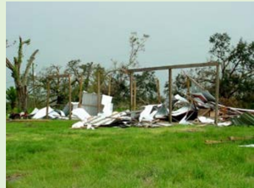
Equipment shed in Hardee County destroyed by a tornado associated with Hurricane Charley in 2004. Photo credit: Doug Mayo
